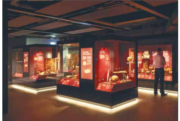
Museum display units often have a system of humidity control within the cases. The Mary Rose Museum has a micro-air-conditioning system for its display cases, each independent of the others, which are in turn connected to the chilled water system. The museum staff set the cases to 55% humidity and 19°C, which is typical for storing organic artefacts © Mary Rose Trust
